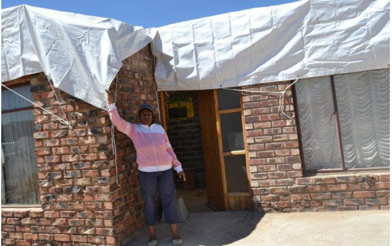
A roofless church ... The whole roof, windows and building structure was blown off the St John church
